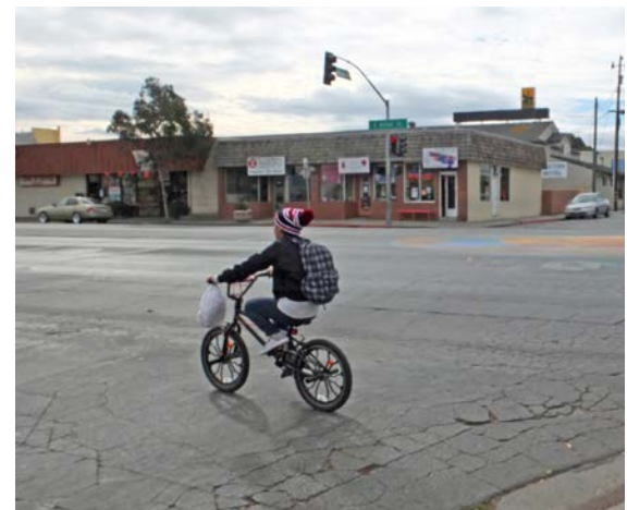
At locations without bicycle facilities, some bicyclists choose to ride on the sidewalk where there is a greater sense of safety. However, this results in conflict with pedestrians using the sidewalk.
