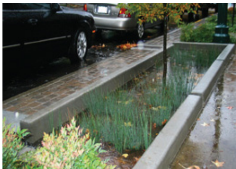
Street Infiltration Planter
